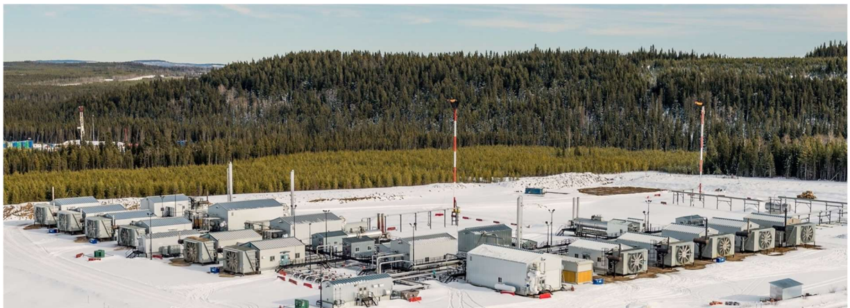
Nosehill Gas Plant, Alberta
