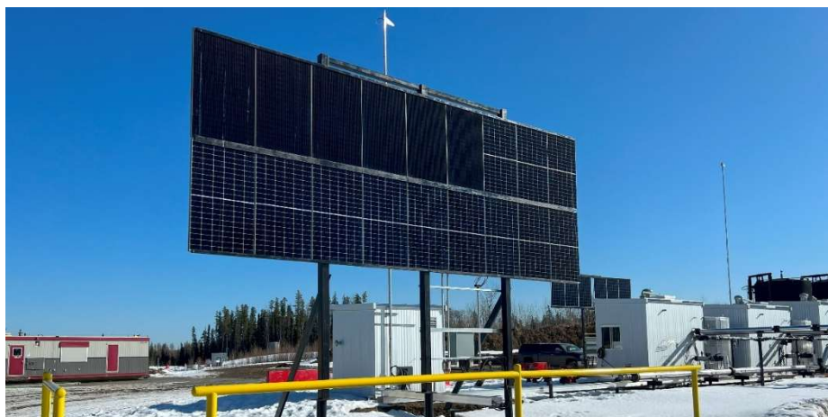
Peyto uses solar panels combined with battery storage to power electrical instrumentation and pumps to reduce Methane emissions.
